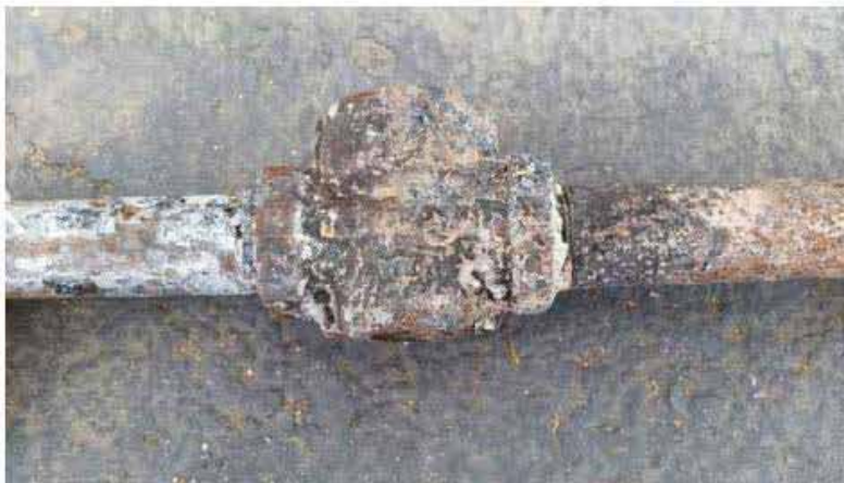
Figure 3. As found service valve body (exterior).
