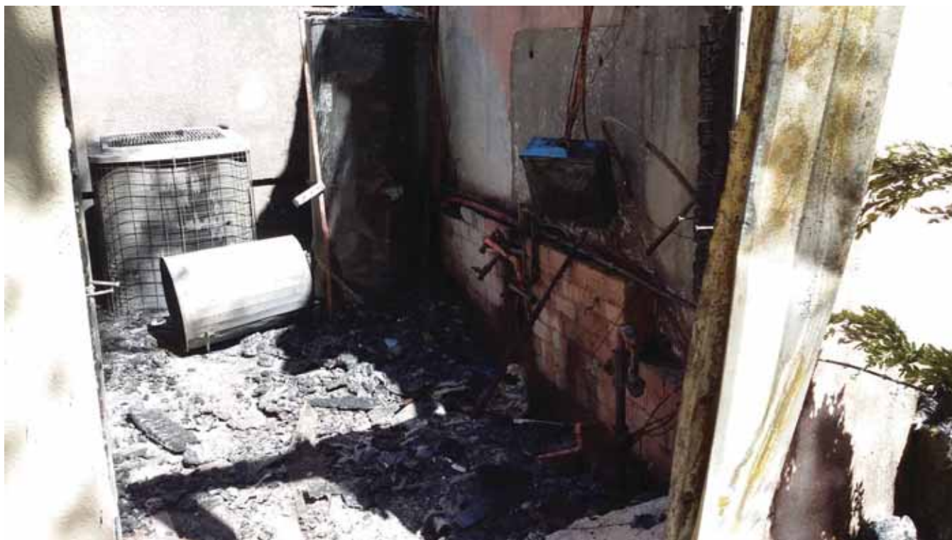
Figure 6: Damage to customer house
