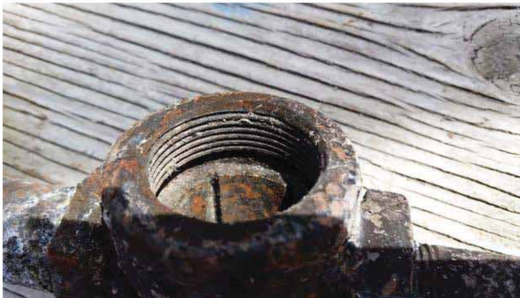
Figure 5. As found service valve body cavity.
