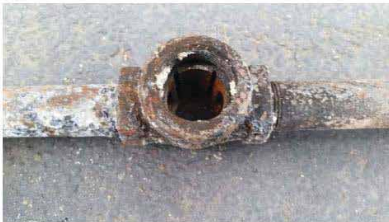
Figure 4. As found service valve body cavity.
