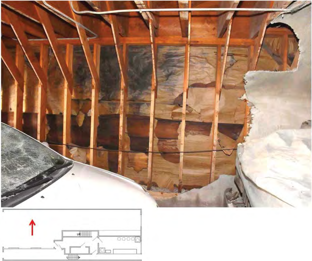
Figure 9. Thermal damage on north wall of garage at incident house. Photo taken by Exponent on December 1, 2017.
