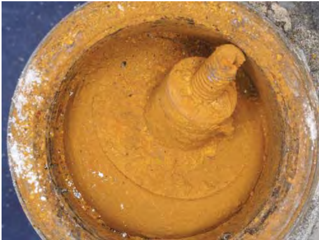
Figure 25. Rubber plug found inside service tee.
