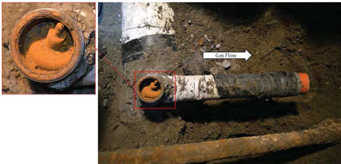
Figure 23. Rubber plug found inside service tee.
