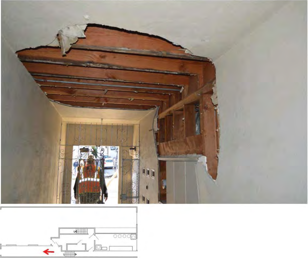
Figure 12. Damage to wall and ceiling in front entryway. Photo taken by Exponent on November 27, 2017.
