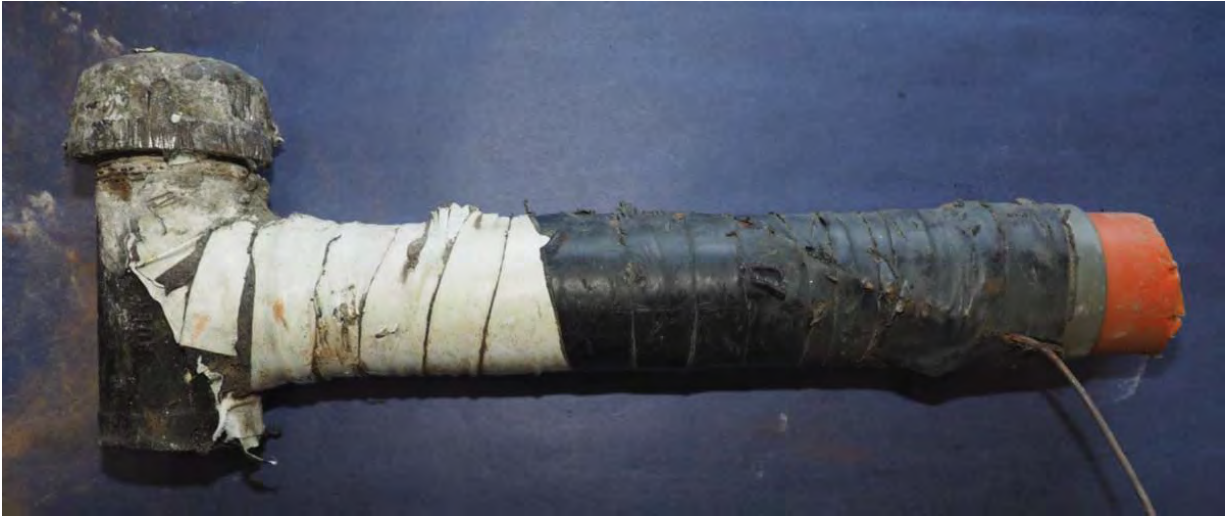
Figure 24. Service tee from at leak location.
