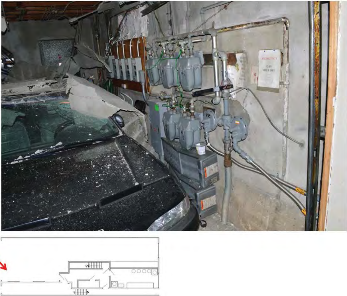
Figure 6. Gas meter set in garage at incident house. Photo taken by Exponent on November 27, 2017.
