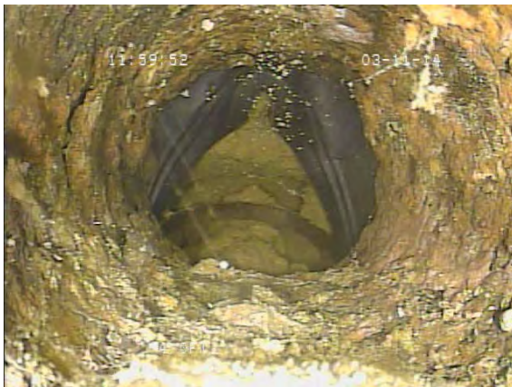
Figure 5. Collapsed main and offset joint
