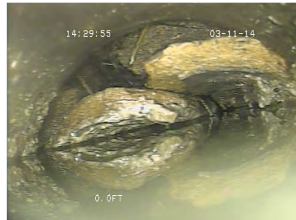
Figure 8. Collapsed main and water in sag
