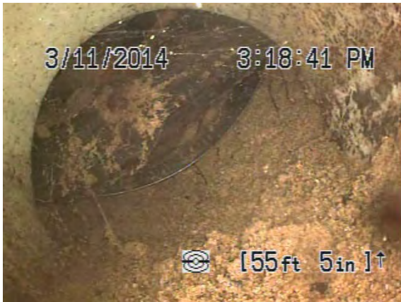
Figure 7. Lateral bend 55 ft. from entry
