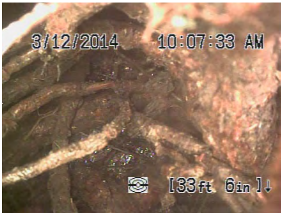
Figure 9. Lateral blocked by roots
