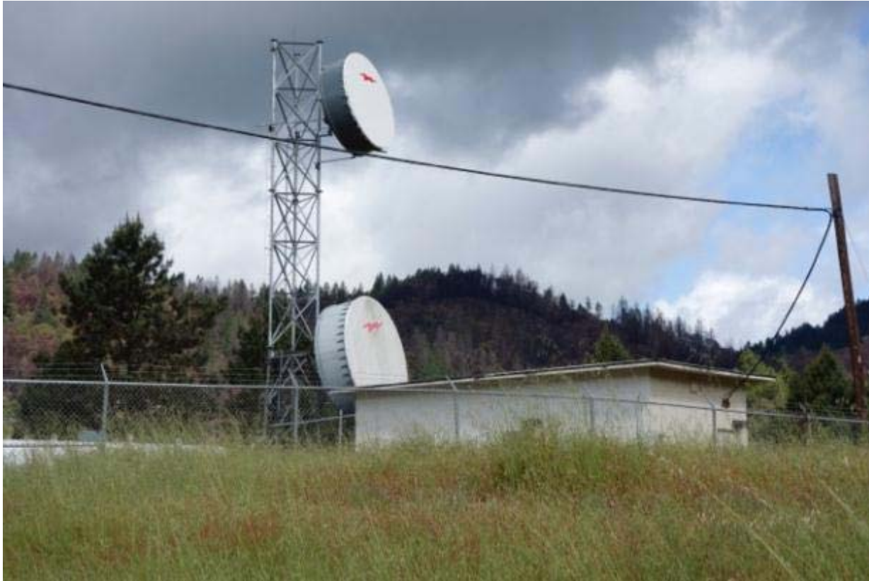
Verizon Microwave Facility, Orleans
