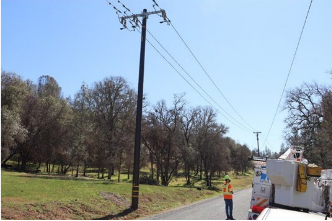
Figure 4: Incident Location and Incident Pole on Iron Horse Rd. in Grass Valley, CA.
