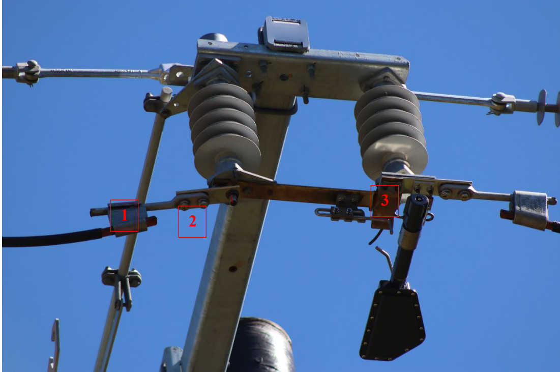
Figure 7: Close-up of new wedge connector (1), bolts on new paddle jumper (2), and switch equipment (3).
